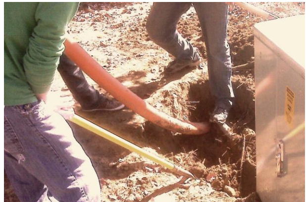
Figure 1: New single mode fiber being run under Park St. to the Academy.
